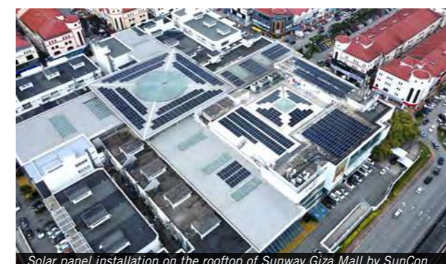
Solar panel installation on the rooftop of Sunway Giza Mall by SunCon
