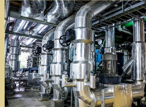
Mechanical, Electrical and Plumbing Services
