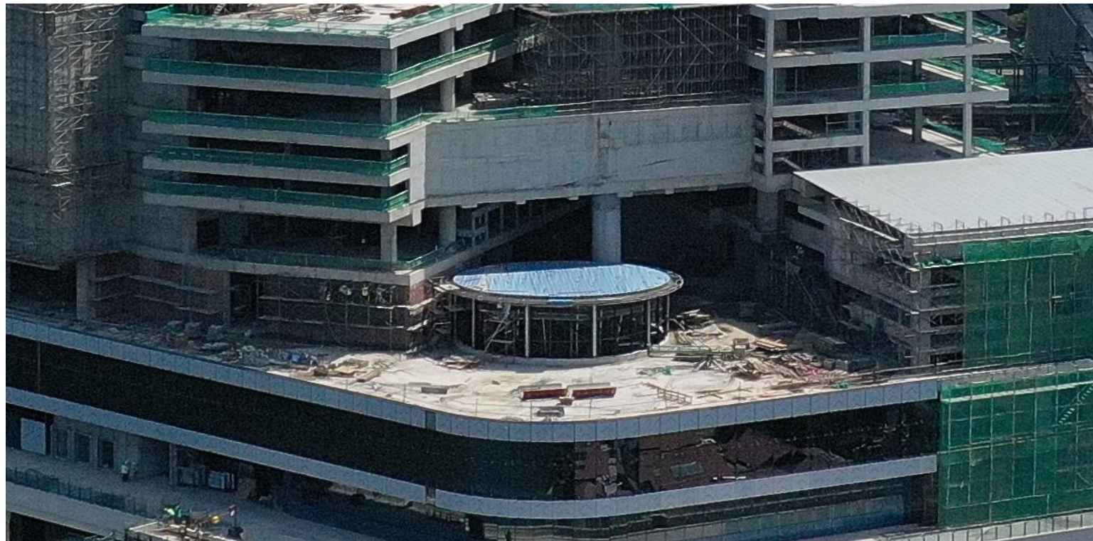
Sunway Square – District Cooling System
