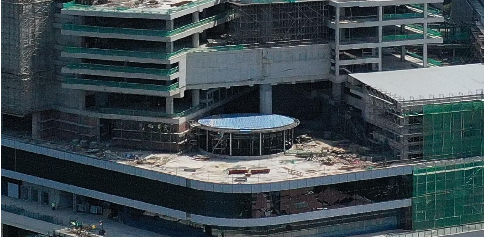
Sunway Square – District Cooling System
