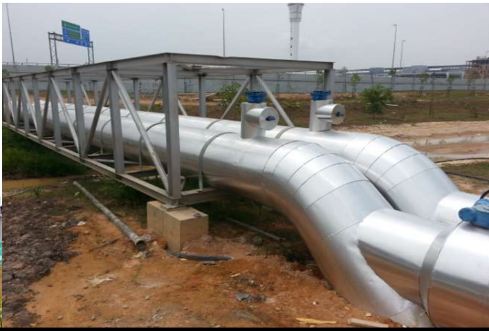
KLIA Chilled Water
