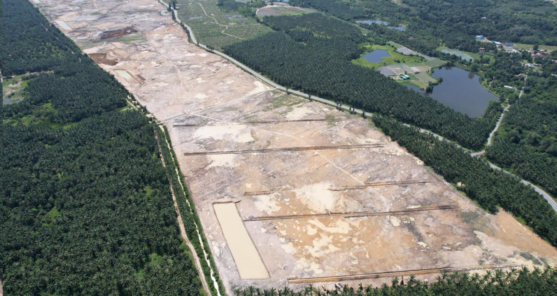
Large Scale Solar 4, Gopeng, Perak (50MW)
