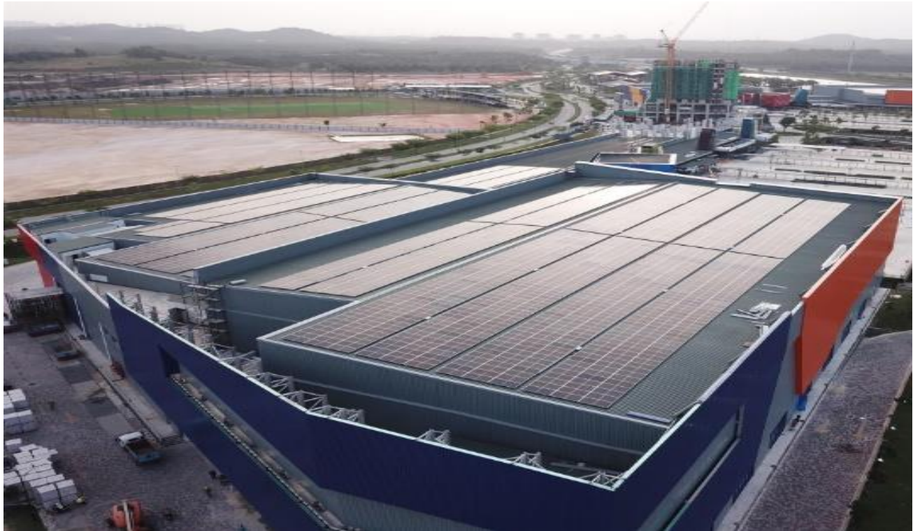
Roof Top Solar – Sunway Iskandar
