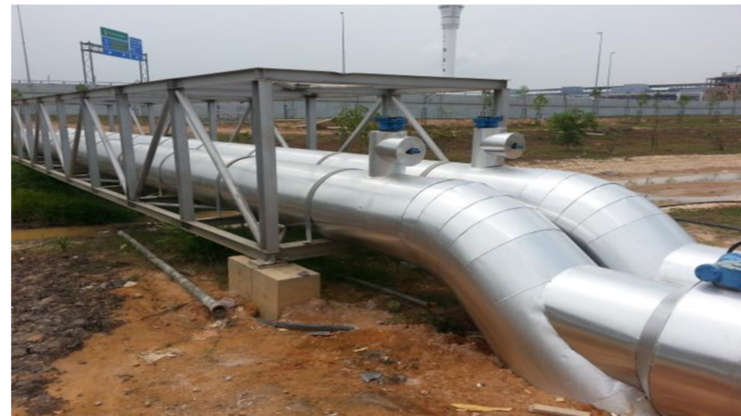
KLIA Chilled Water
