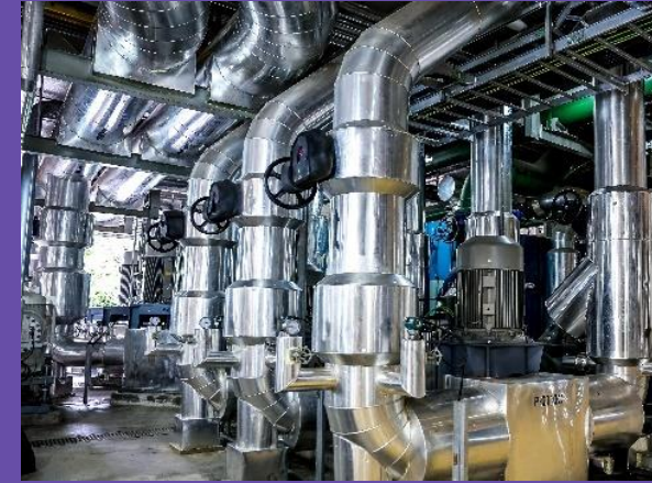
Mechanical, Electrical and Plumbing Services
