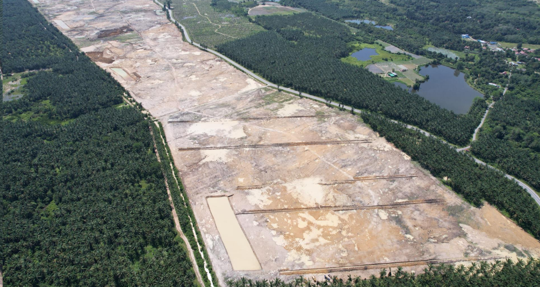
Large Scale Solar 4, Gopeng, Perak (50MW)
