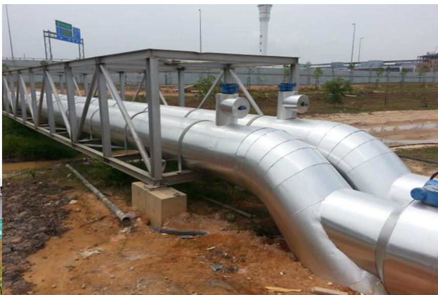
KLIA Chilled Water
