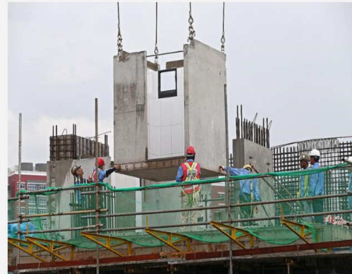
Prefabricated bathroom units are assembled with finishes in a factory before it is transported to a construction site for installation. PHOTO: LIANHE ZAOBAO
