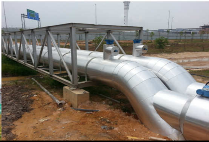
KLIA Chilled Water
