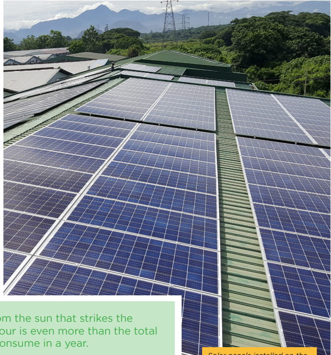
Solar panels installed on the rooftop of one of i2 Energy's client in Selangor
