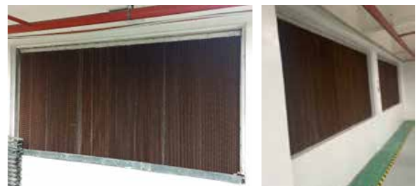
Water cooling system in operation floors
