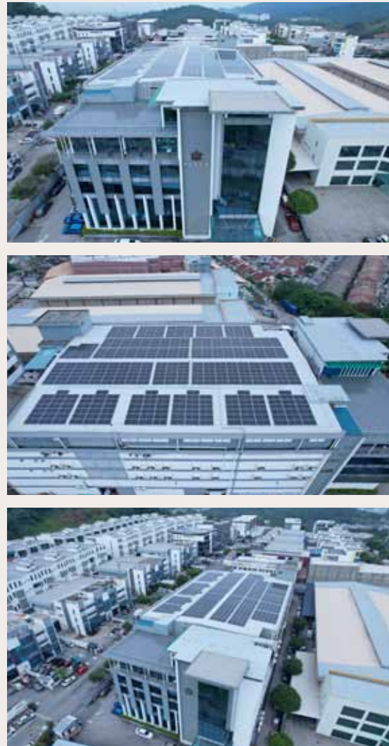
Figure 2: Completed solar PV system on the rooftop of our manufacturing facility
