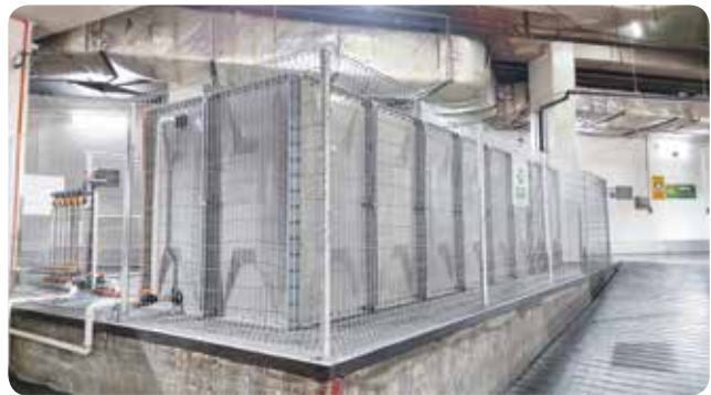
Rain Water Harvesting located at Pavilion Kuala Lumpur Mall.
