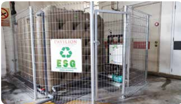
Condensate Harvesting located at Pavilion Kuala Lumpur Mall.
