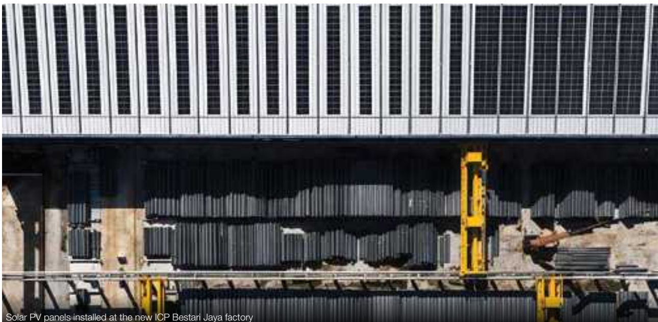
Solar PV panels installed at the new ICP Bestari Jaya factory
