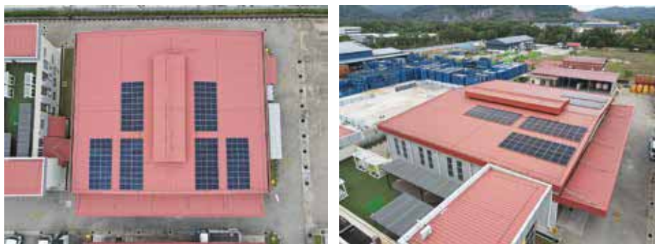
Solar PV installations at Hextar Kimia's facility in Kemaman, Terengganu in FY2025, supporting renewable energy adoption and lower-carbon operations.
