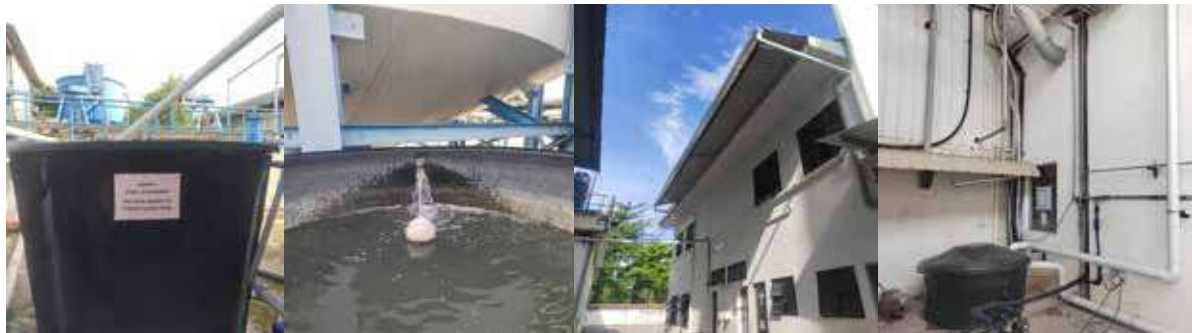
Rain water harvesting at Hexcare's glove production plant in Ipoh, Malaysia
