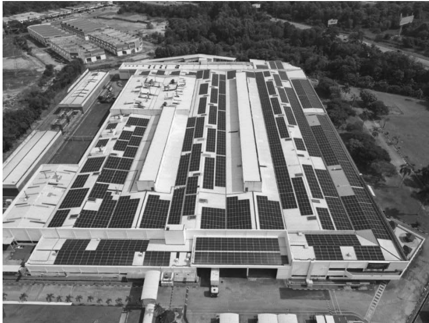
A 3.90 megawatt peak solar PV system installed at an industrial building in Nilai, Negeri Sembilan
