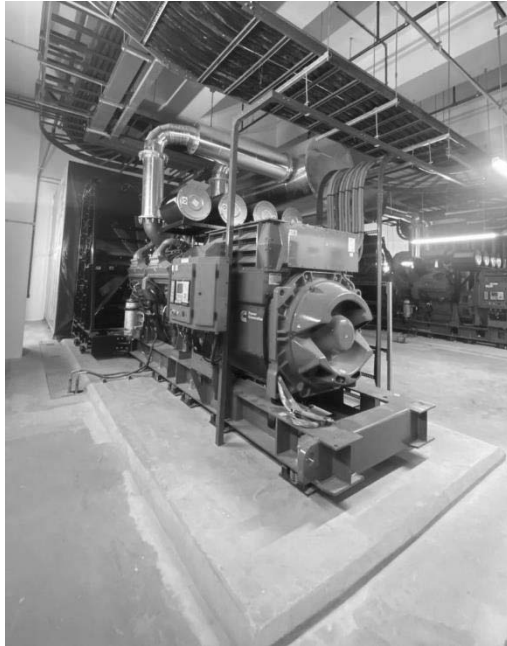
An installed generator set for a diesel generation system installed at an industrial building at Batu Berendam, Melaka
