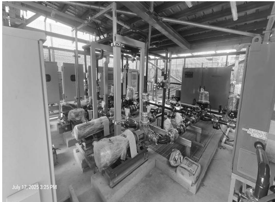
Installation of a pump house and PLC system for a diesel generation and fuel distribution system for a data centre in Cyberjaya, Selangor.
