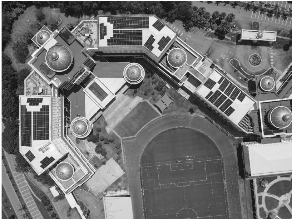
A 0.48 megawatt peak solar PV system installed at a commercial building in Seremban, Negeri Sembilan
