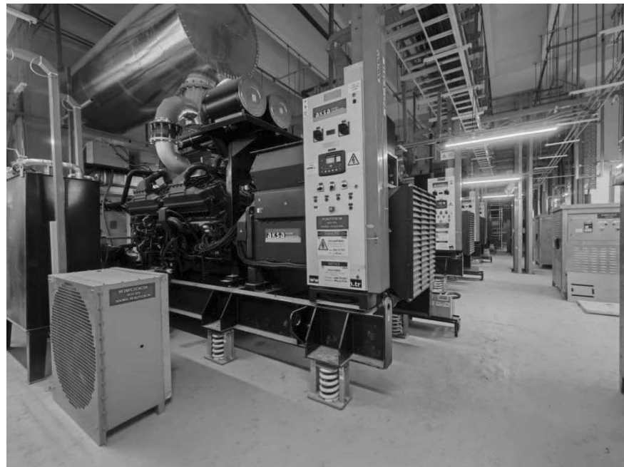
An installed generator set and PLC system for a diesel generation system installed at an industrial building at Kawasan Perindustrian Bayan Lepas, Pulau Pinang
