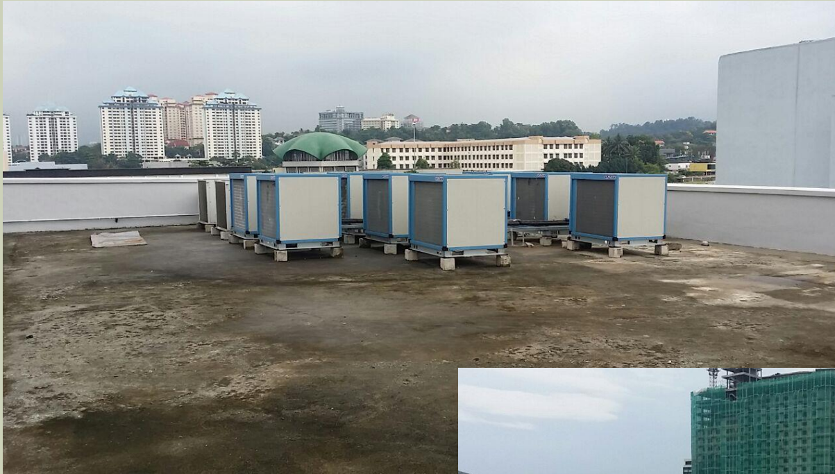
New environmentally-friendly R410A air-conditioning system cluster on rooftop
