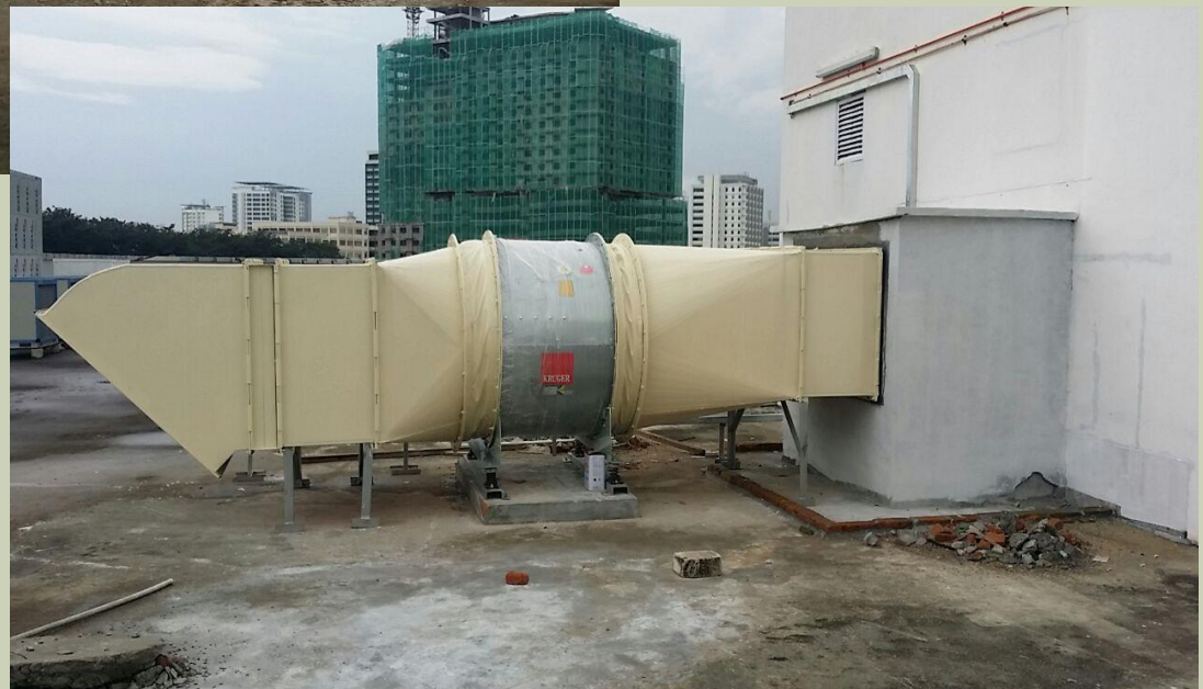
New smoke spill system complying with Bomba requirements
