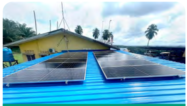
Solar panel at Ladang Sungai Tenegang, Sabah.
