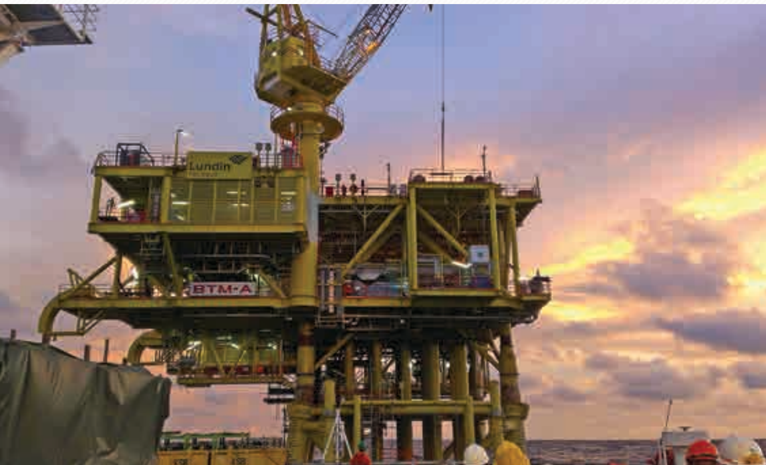
• Hook-Up & Commissioning - Materials transfer in progress at Bertam-A Platform for Lundin Petroleum
