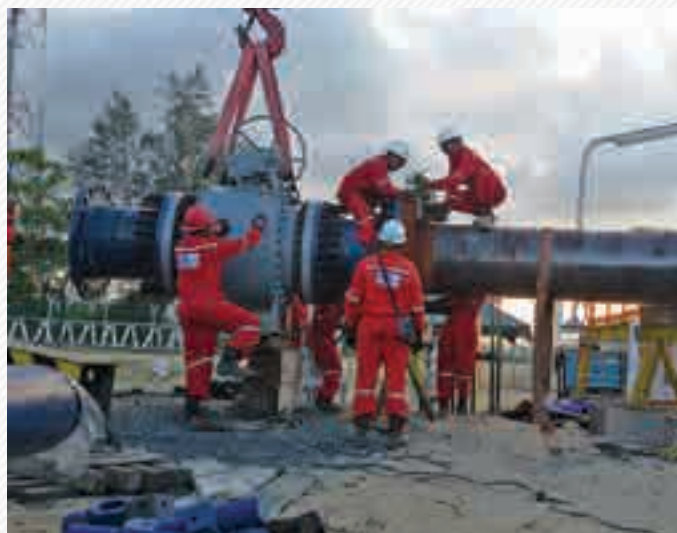
• EVA project for the North Malay Basin gas pipeline - Pre-commissioning work in progress
